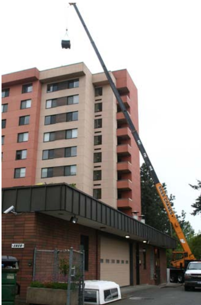
GREEN HOUSING: Construction workers for Hytech Roofing, Inc. install solar panels on the Lincoln Square apartment complex roof Wednesday, May 25. Photo by Sarah C. Richardson | THE WESTERN FRONT
